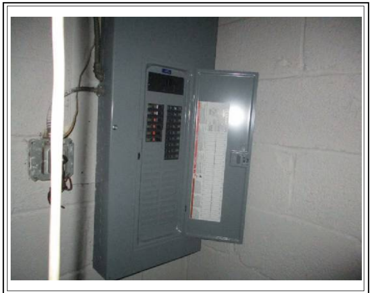
Basement - Electric Panel
