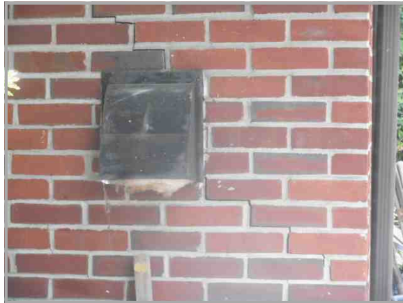
Some Minor Settlement Cracks
