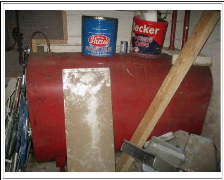
Basement - Oil Tank
